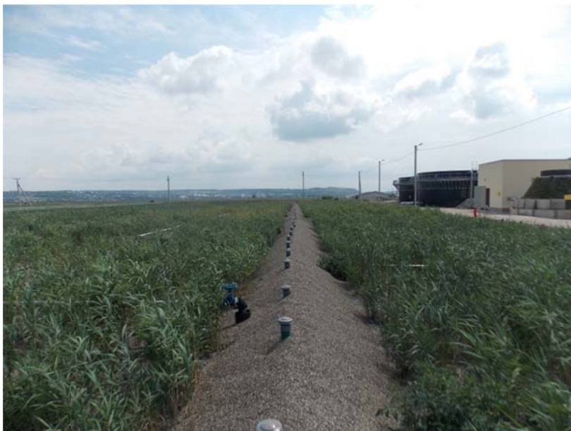
French Reed Beds with pre-treatment building and equilisation tanks in the background. Credit: Riccardo Bresciani
